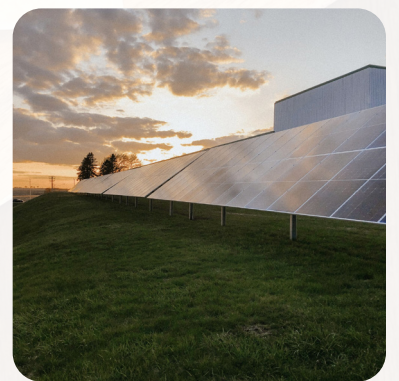
Driftless Provisions completed its 800 square foot solar drying chamber this past March.
